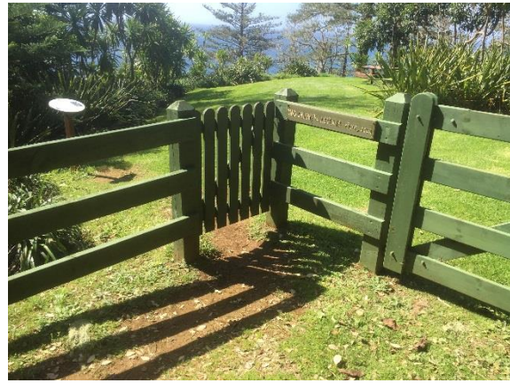
Figure 13. Pedestrian access to a second picnic area is through a timber gate. Note the condition of the sign.
