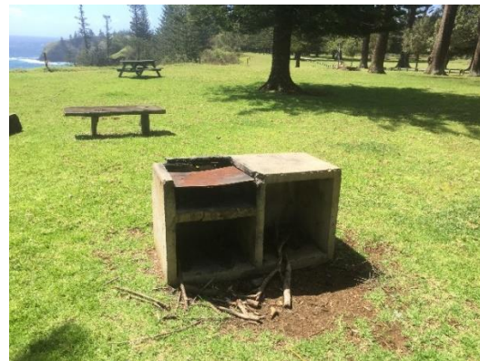
Figure 10. Both Barbeques have been well used and are in disrepair
