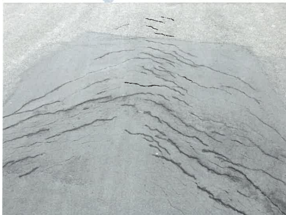
Figure 2 Photo example of slippage cracking at the 11 turning end
