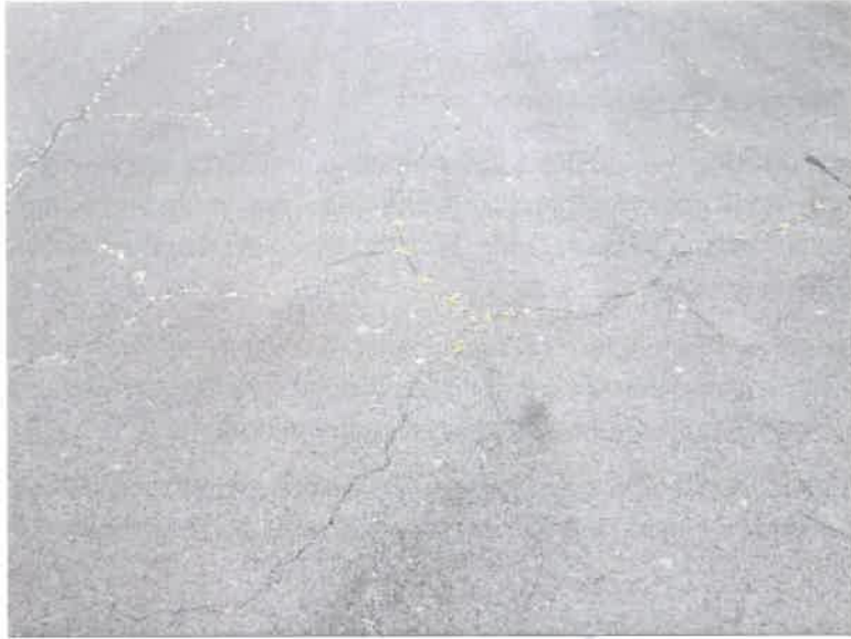
Figure 6 Photo example of block cracking at Norfolk Island
