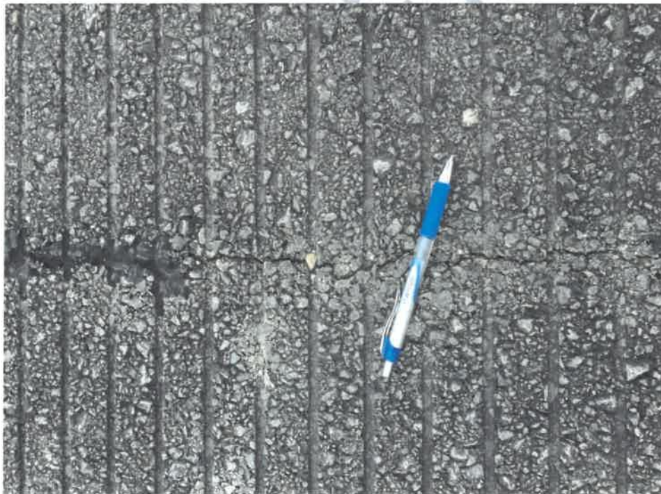
Figure 4 Photo example of an open and unsealed low severity longitudinal crack at Norfolk
