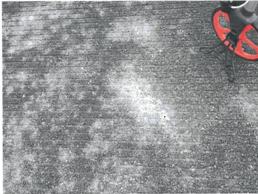
Figure 5 Photo example of white staining at Nelson Airport
